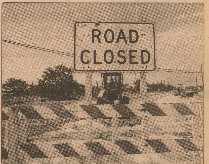
Street repairs in progress — Crews from Seidel Construction began street repairs on West Avenue last week. Paving and repair work will continue through the summer in the north west and north parts of town.
