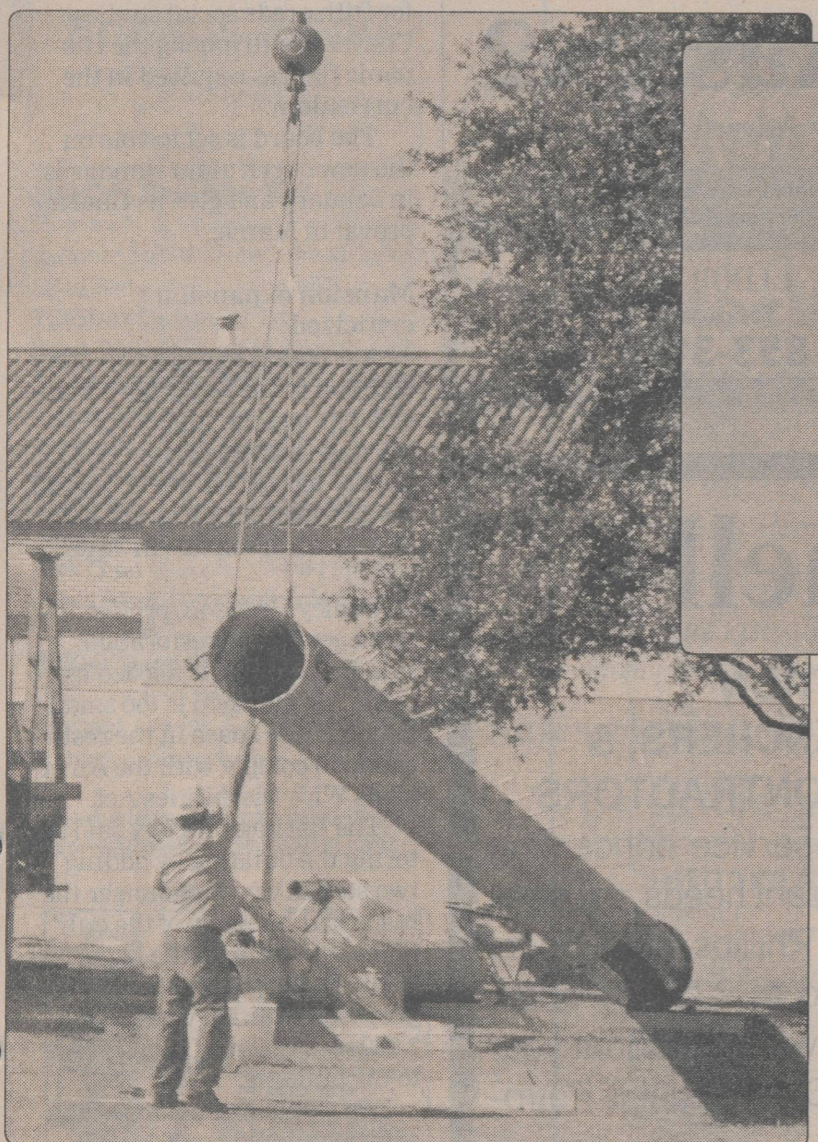
Workers erected a tower last week on the Elementary School campus. The tower will support a microwave antenna that will provide the school with a wireless connection to the Region XV offices in San Angelo. The connection will also provide the school with a boost in speed for its Internet service.
