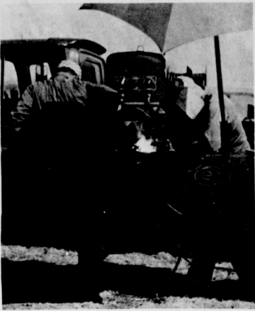
WELDING JOINTS —Joint after joint of pipe, approximately 60 feet in length, are being welded together to form a line across the county. It is being put down by Natural Gas Pipeline of America. Welder Charles Ellard has almost completed this section for inspection. Inspector of the welding operation is Art Pfeiffer.
