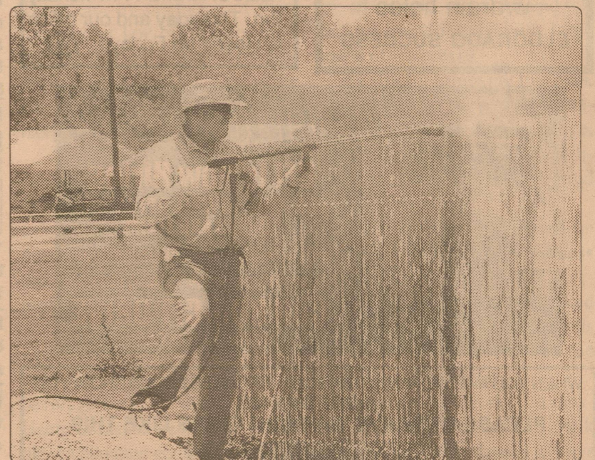
The work goes on — SCISD employee Oscar Martinez used a pressure washer to strip paint from a fence at the bus barn last week. Several maintenance projects are being carried out during the summer months.
