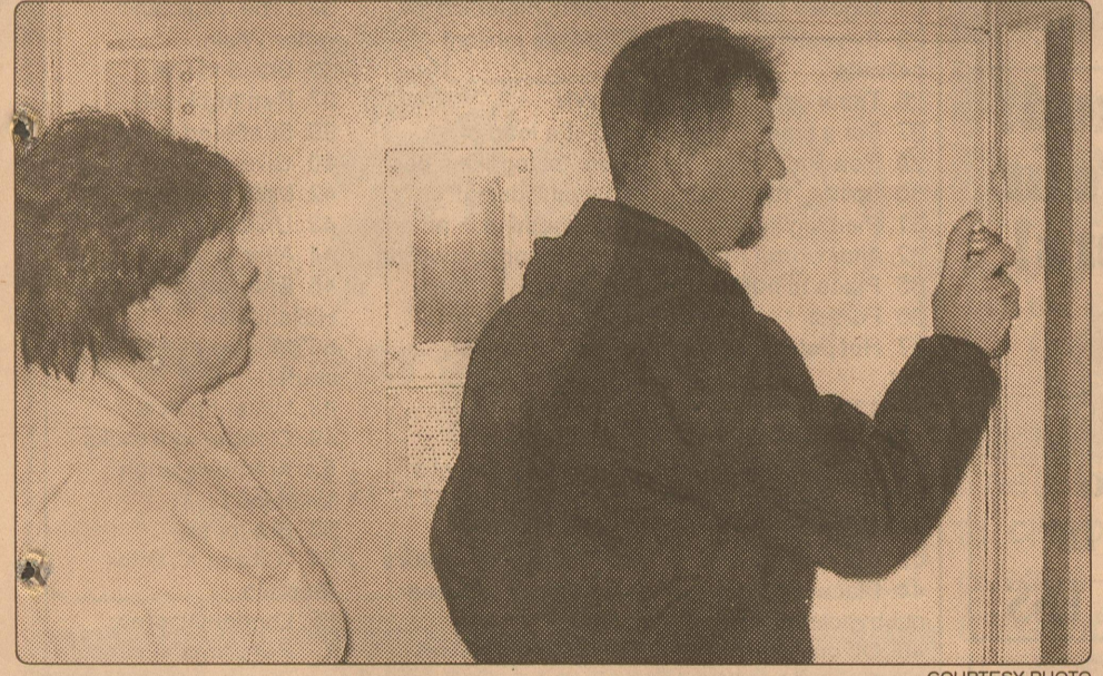
Jail inspection — Jail Administrator Lesa Martinez looks on as Jail Standards Inspector Russell Biehle sprays an aerosol mixture into a plumbing closet to test a smoke detector.
