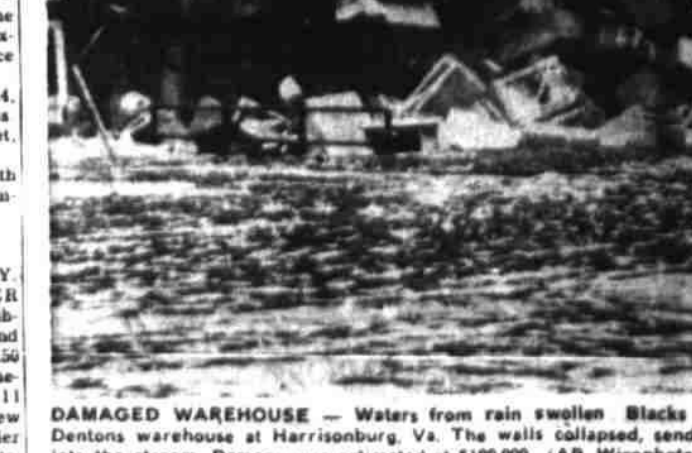
DAMAGED WAREHOUSE — Waters from rain swollen Blacks Run undermined two walls of Dentons warehouse at Harrisonburg, Va. The walls collapsed, sending furniture and bedding tumbling into the stream. Damage was estimated at $100,000. (AP Wirephoto)
