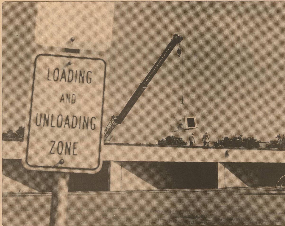
Heavy lifting – Workers installed new air conditioning units this week on the roof of the Elementary School in preparation for the beginning of school next Monday.
