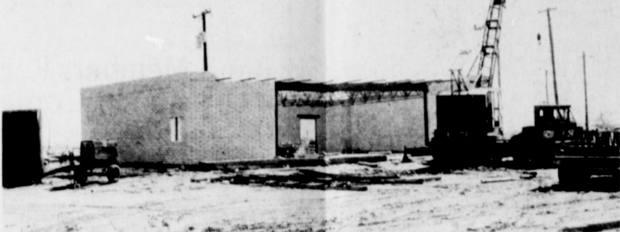
With a let-up in the wintry weather, construction has been progressing on the building at the corner of Rowe Street and the eastbound lane of Interstate 40 that will house a Wal-Mart convenience store. The Wal-Mart chain is owned by Jerry C. Wilson of Pampa.
