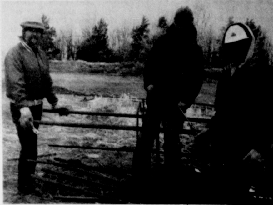
DESPITE FREEZING TEMPERATURES these J. D. Abrams Construction Co. workers continue with their work building part of the undergirding for an overpass. [Photo by Linda Haynes]
