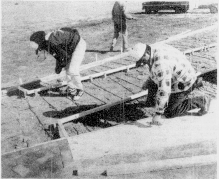
Workers prepare forms to pour concrete, and lay brickwork in preparation for the third Station of The Cross at the Cross of the Plains just west of Groom.
