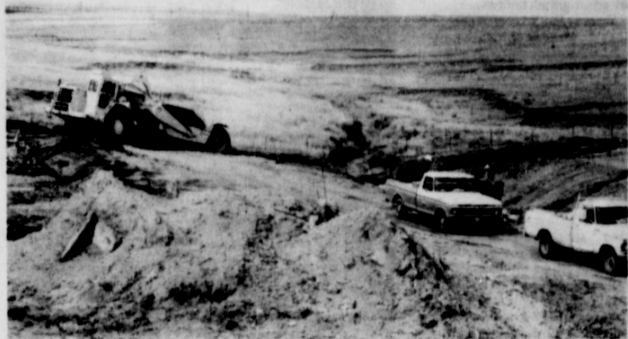
CONSTRUCTION ON I-40 between McLean and Alanreed got underway last week. The new four-lane highway will not be completed for several months. [Photo by Linda Haynes]
