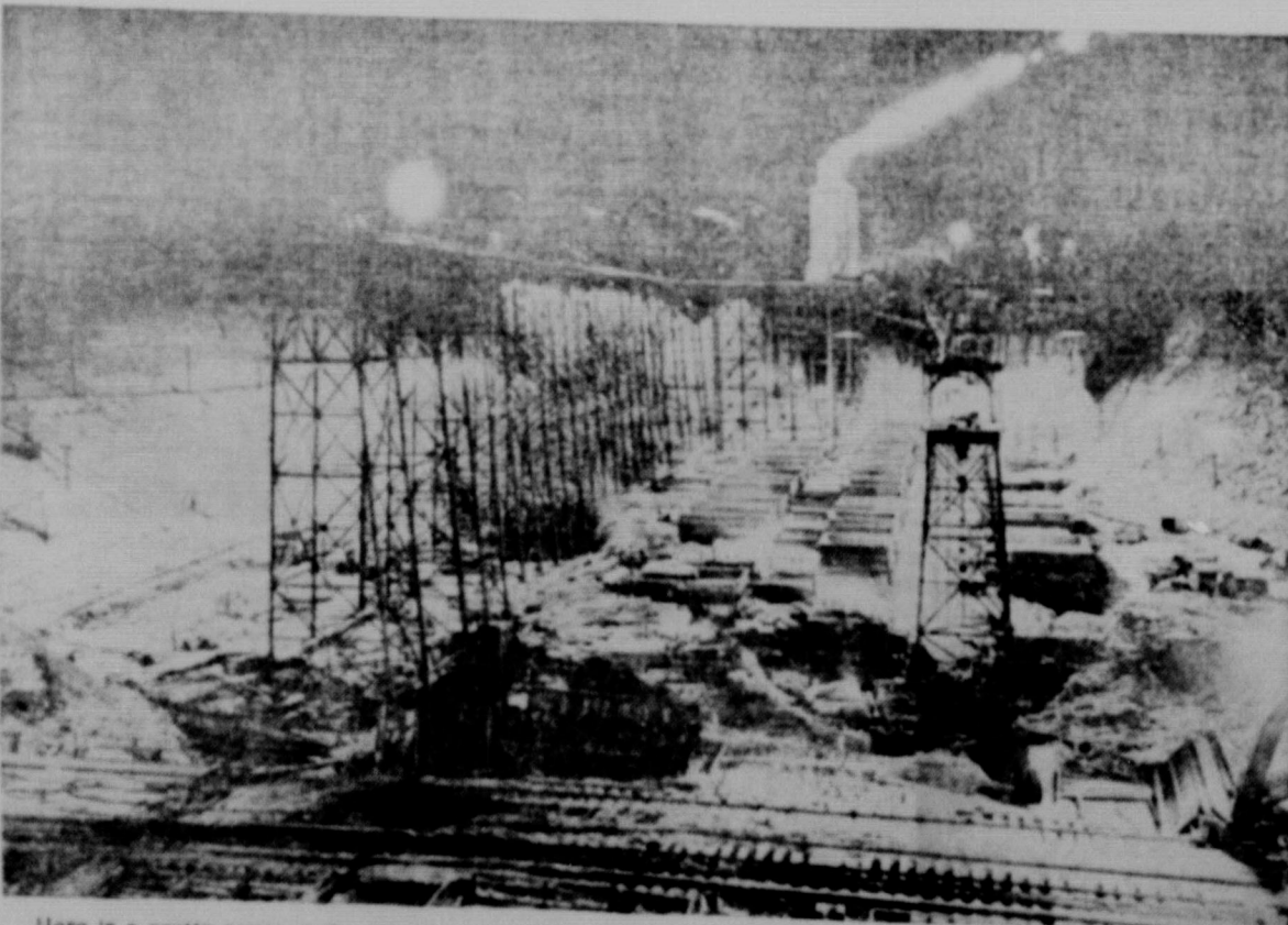
Here is a pretty scene at the site of the federal government's huge power project on the Columbia river as work is rushed to complete the Grand Coulee dam, to harness the river and to supply electric energy to the countryside. Nightfall does not bring a halt to work, as banks of lights illuminate the excavation.
