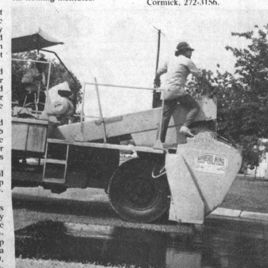
SEALCOATING OF CITY STREETS--It's a bother and hard to get off vehicles, but local residents are happily adjusting to the sealcoating of city streets, which will prevent chug holes that provide a lot of "wear and tear" on tires and vehicles. Sealcoating can be found all over the city at this time.
