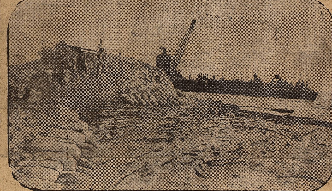
Two scenes in the struggle waged by southern dyers to keep "Old Man River" within his boundaries are graphically portrayed here. Workmen are trying to save the levee at Mounds Landing, 18 miles north of Greenville, Miss., where the 1927 levee break flooded Greenville. At the top, the Jadwin system of levee building is shown in its first real test. Sand, earth and silt is pumped from the river bed to build the levee. Many skeptics have held that such a levee would never hold, but it has held so far. The lower picture shows a bad slough which has been stopped by the use of sand bags and the sinking of a willow mat. The battle to save the levee will be decided within the next two weeks.
