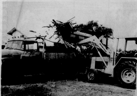
AND AWAY IT GOES -- Old boards, tree branches and roots, used cartons, you name it and if it was unsightly or tended to tarnish the image of the neighborhood in the vicinity of 18 South Barkley it doesn't anymore. As can be seen, it was all pushed into a pile and loaded aboard this truck to disappear as Spearman cleans up for the future.
