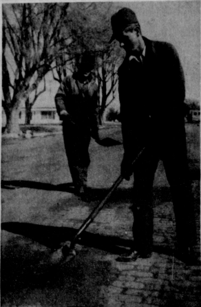
REPAIR WORK -- Jimmy Joe Bonham and Frank L. Nelson, nearest camera, are employed by Texas Highway Department and the Gruver residents were busy filling potholes in Spearman recently.
