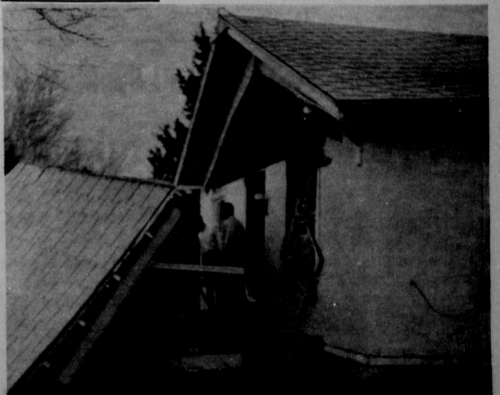
LIVING ROOM - This is the living room of Mrs. Inez Kirk's home after a gas explosion ripped the house apart. The furniture was upset and covered in inches of insulation from the ceiling of the house.
