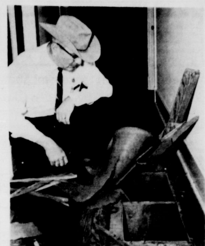
HOLE IN THE FLOOR—Sheriff J. D. Spray examines hole made above First State Bank vault.
