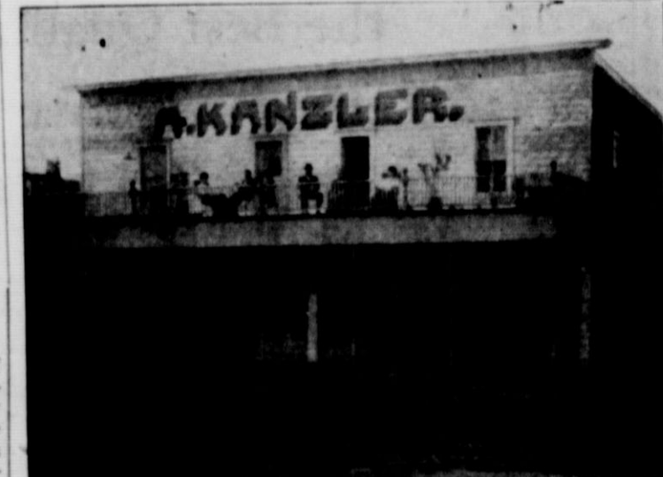
The Kanzler building is being torn down. One of Matador's first buildings will soon pass into history, as workmen recover material of value in the structure erected in 1901. The above picture, courtesy of Mrs. W. W. Moore, shows the building shortly after its erection. Seated on the balcony are Mr. and Mrs. P. A. Sandlin and daughter, Mae, Mrs. Sandlin's parents, Mr. and Mrs. A. Kanzler, and Miss Mae Kanzler who later married F. A. Loveless. Top floor of the building was used for offices and apartments. The balcony was removed years ago. The property was acquired this year by J. M. Jackson from J. K. Crews, under agreement that the building, which had become a "firetrap", be removed.
