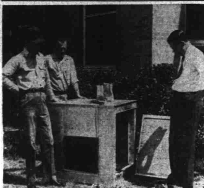
COMFORT FOR OTHERS —W. C. Jones, Big Spring, left, talks over installation of the air-conditioner he built for the Texas & Pacific employees hospital in Marshall with C. F. Spencer, chief of maintenance at the hospital, and Louis Richardson, chief clerk. Jones, T&P train baggageman, was a patient in the hospital last summer and promised the air conditioner to Dr. C. McCurdy at that time. Last week he made good, delivering the unit for installation. (Marshall News Messenger Photo by Bob Burns.)
