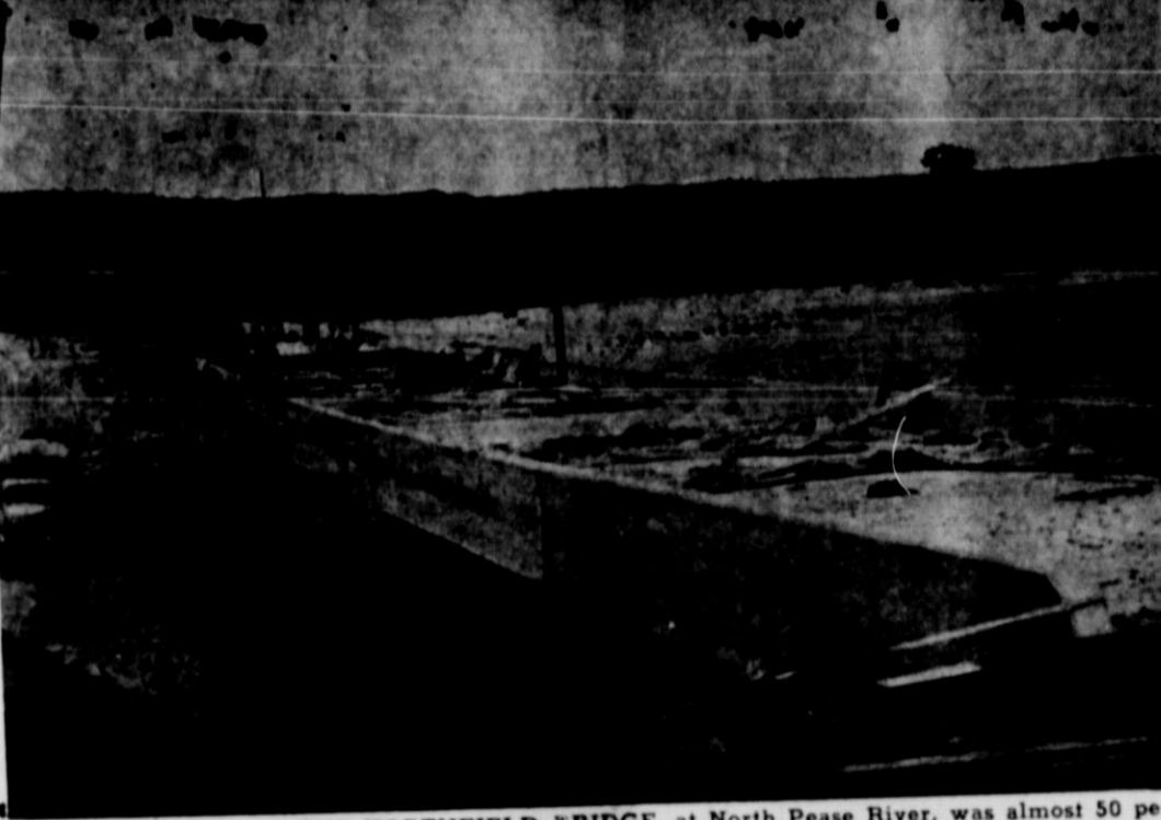
CONSTRUCTION OF THE NORTHFIELD BRIDGE, at North Pease River, was almost 50 percent completed last week. Concrete was being poured near the middle of the bridge which is an estimated 520 feet long. The finished north end of the bridge is shown in the above photo. The new bridge is being built in the exact location of the old wooden bridge. —Childress-Index Photo-Engraving.
