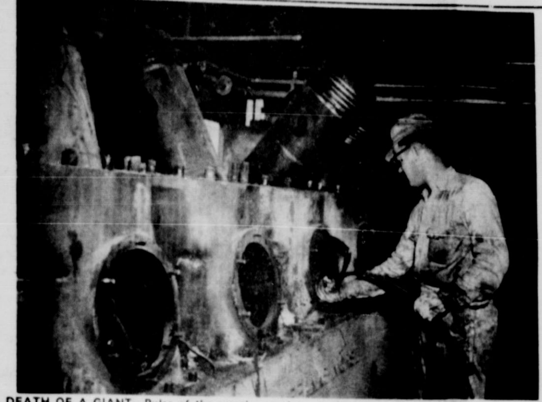
DEATH OF A GIANT —Pulse of the massive engine at the West Texas Utilities Company plant in Matador is silenced forever as workmen cut the 60,000-pound giant into pieces and hauled it away as scrap metal. The diesel was moved here from McCamey in 1931.
