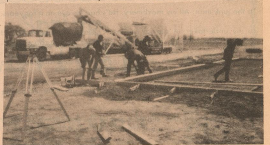
Foundation being poured Tuesday, April 2nd at the site of Quail Pipe Corporation, Roaring Springs, Texas. The factory will initially employ 25 people.
