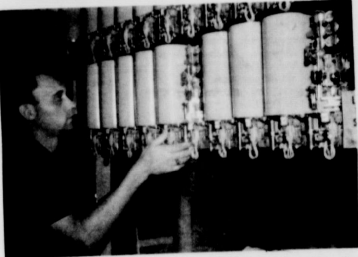
SILENT SWITCHBOARD and Chief Operator Mrs. Dorothy Knight Wednesday morning after the cutover to dial telephones in Matador. District Plant Supervisor J. L. Bates, top in center picture, and Lineman Gene Collier, pull the strips of insulation away that made every telephone in Matador automatic dial. In lower picture District Manager W. L. Frazier checks one of the complicated selector switches in General Telephone's new installation on Lariat Street. —Photos by Doug Meador
