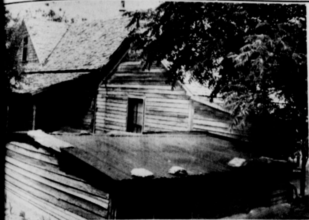
PHOTO BY DOUGLAS MEADOWS OLD HOUSE is getting shaky . . . this old house is badly worn . . . this old house has shingles . . . words from the song, "This Old House," have a sentimental meaning for Mrs. Chas. Keith. They are in the process of replacing the old original homestead grandsons, Mr. and Mrs. P. A. Cribbs, Motley County pioneers, with a modern home. Late Mr. and Mrs. Cribbs first lived in the dugout, shown in the foreground, which had a place originally, but later removed. Mr. Keith's parents, the late Mr. and Mrs. D. C. Keith lived there a number of years, and the Chas. Keiths have resided there for 15 years.
