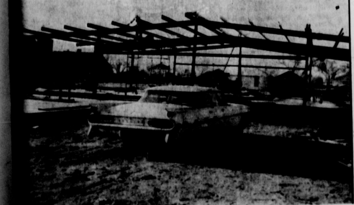
SCENE CHANGING — The above picture made late Saturday of El Matador restaurant and station is changed today, with the roof completed and side walls going into place. House at upper left is home of Mrs. G. E. Hamilton. Interior work is also underway in the building. Concrete at left of automobile is island for filling station pump.
