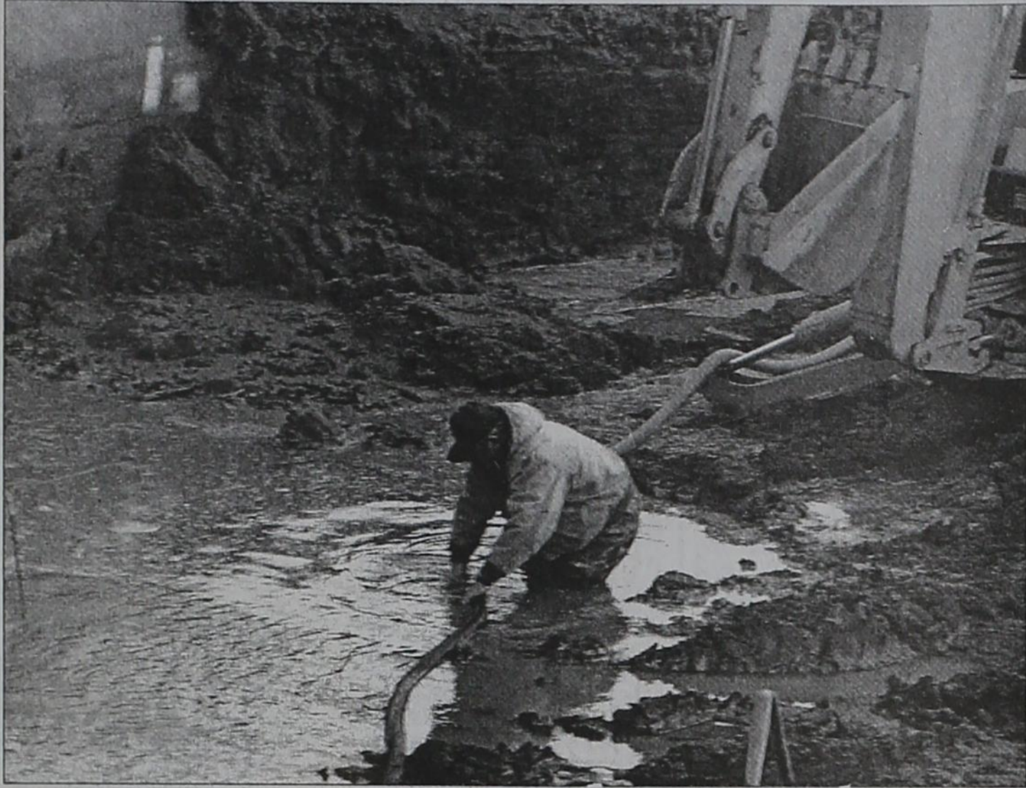
BIG LEAK! Matador City Water Superintendent, Steve Barton, is up to his knees in water trying to fix a big leak in a main city water line, last Wednesday night. The line was accidentally broken while preparations were being made for the Motorcycle Race course. The entire city was without water for 3-4 hours, before city employees repaired the line.
