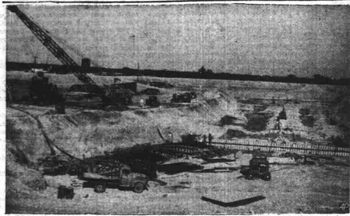
STARTING THE CONCRETE JOB - The pouring of the first of nearly 50,000 yards of concrete has started on the outlet works of the North Concho Dam just northwest of San Angelo.
