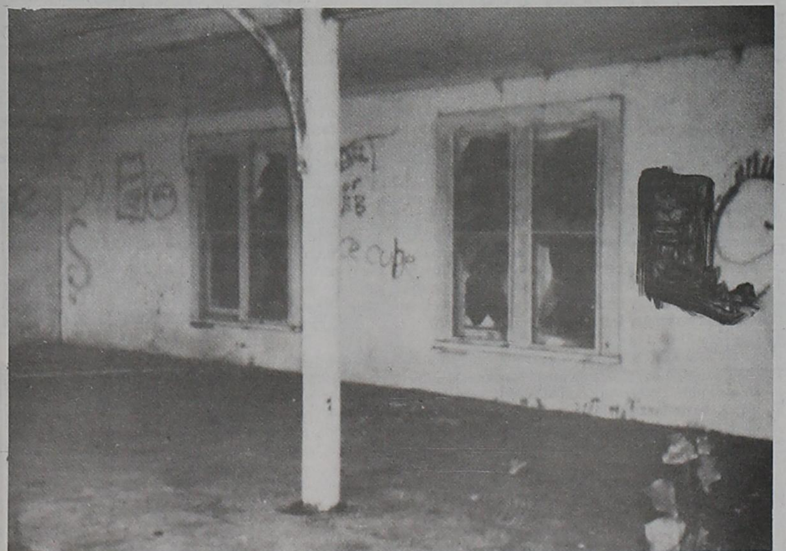
VANDALISM — According to reports from Motley County Sheriff, Jim Meador, the Motley County 4-H building has been vandalized on different occasions resulting in 13 broken windows and profane graffiti spray painted on the outside walls of the building. 4-H leaders have stated that this property belongs to the Motley County 4-H club and anyone caught on the property will be prosecuted to the fullest extent. Sheriff Meador stated that a reward is being offered for information leading to the arrest and conviction of the person or persons responsible for these acts. (Due to profanity, some of the picture has been blacked out)
