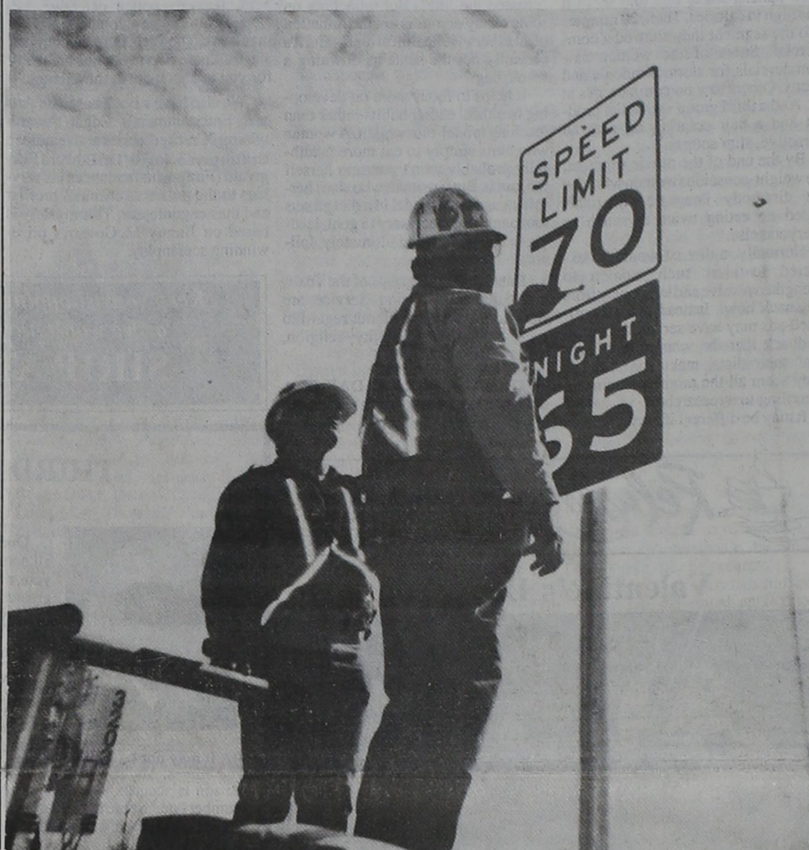
NEW SPEED LIMIT SIGNS — Texas Department of Transportation employees, Randy Martin, left, and Vaden Hays, begin putting up new speed limit signs in Motley County on Tuesday. They expect to complete installing the new signs by the end of the week.
