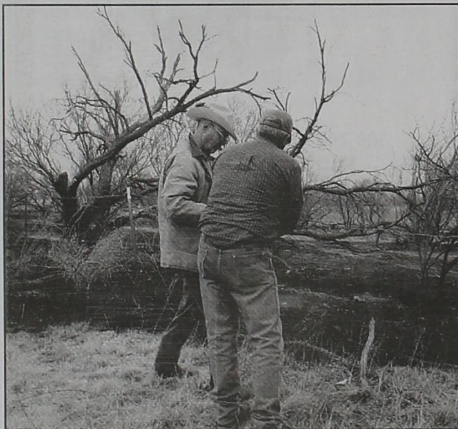
Pictured is Ed D. Smith and Roy Hobbs working on fence on property located about 1/2-mile north of Bob's Oil Well on State Hwy. 70. Roy had cattle on the property that escaped the fire storm. photo by Carol Campbell
