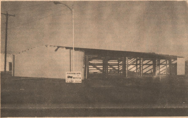
NEW FIRE STATION -- Members of the Matador Volunteer Fire Department are continuing the construction of a new fire station in Matador. The building will house all of the present equipment in one location and will cut down response time when answering a fire call. Firemen hope to have the building completed and in use as soon as possible.
