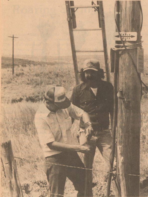
WORKING ON LINE -- On Tuesday, September 14, as a result of a major thunderstorm in the Crosbyton/Matador area, General Telephone's major toll cable facilities on Highway 82 East were struck by lightning, putting customers out of service in Matador and Rearing Springs. Working on a 24 hour commitment, General Telephone employees cleared the trouble at 2:30 p.m. on Wednesday, September 15. Pictured are John Spivey (left), Cable Splicer in Ralls and Alex Zepeda, Cable Splicer in Idalou.
