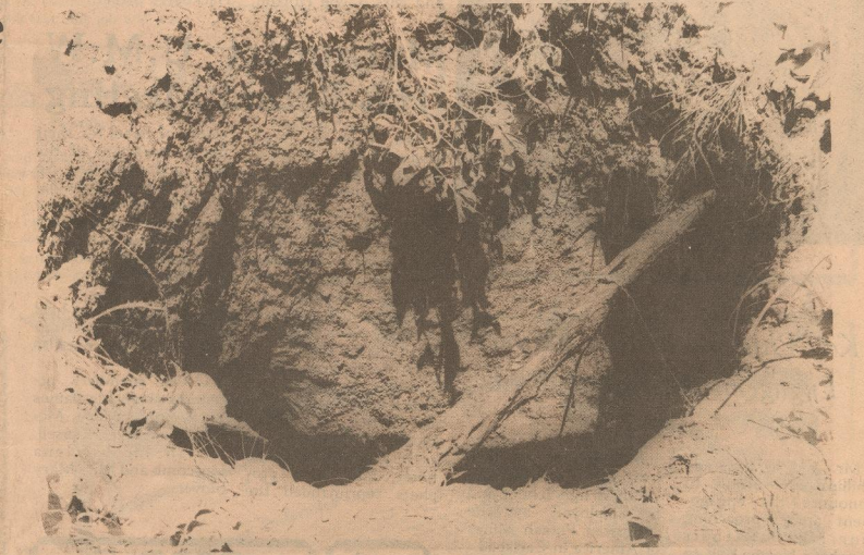
MATADOR SINKHOLE -- When Bill Durham went to his backyard last Thursday to check his garden he discovered a sink hole in the center of his beans. The hole is about ten feet deep and measures five or six feet across. It is believed the hole was probably once a cesspool.
