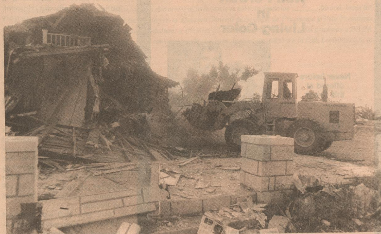
COUNTY AIDS IN CLEANUP - The former home of Gerald Pipkin is being torn down by county equipment in a continuing effort to clean up the destruction left by the May 1 tornado. (Photo by Mary Renfro)
