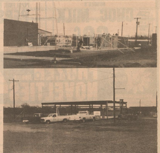
Signs of the Time-Construction is underway around the square in Matador. Pictured above is the new United States Post Office being built west of the present P.O. Below is the construction of the Matador Senior Citizen Center which is north of the courthouse.
