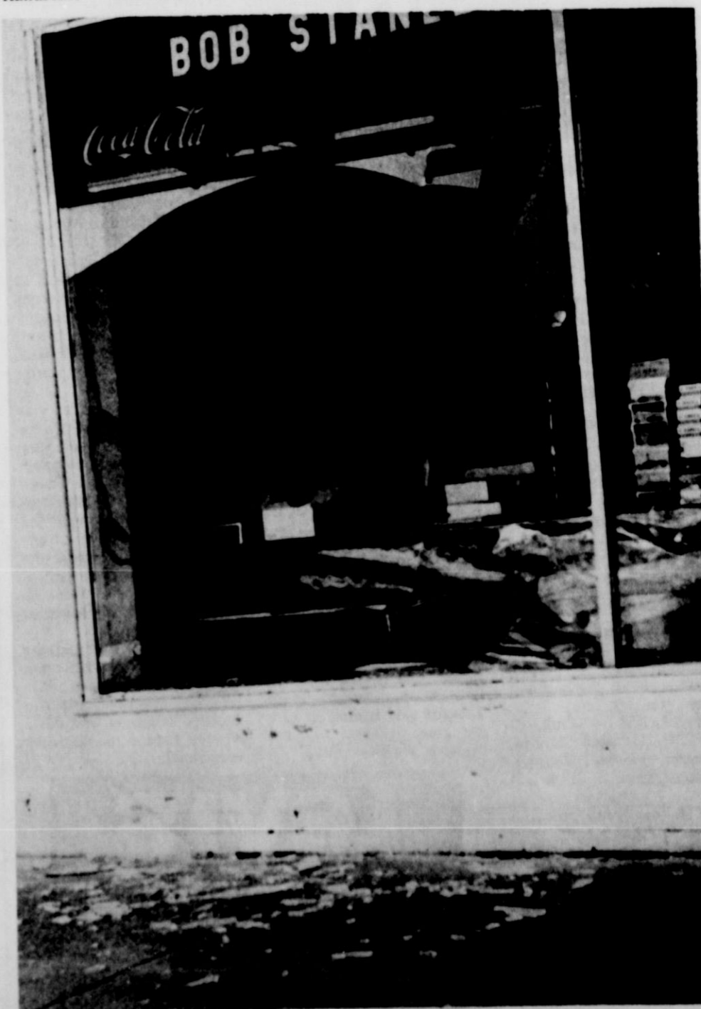
SMASHED WINDOW - Plate glass window on the east front side of Bob Stanley Pharmacy was smashed between midnight Thursday and dawn Friday, by vandals who stole an amount of drugs and money.
