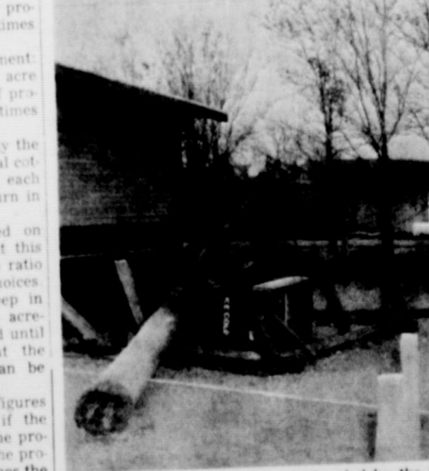
TIMBER — 60-foot light pole toppled by the high wind November 26 at Burleson Field. The poles were installed approximately 30 years ago and decay caused this one to give away when hit by the wind. Freddie Welling, manager of West Texas Utilities Co. here said another pole is decayed and will need to be treated or replaced.
