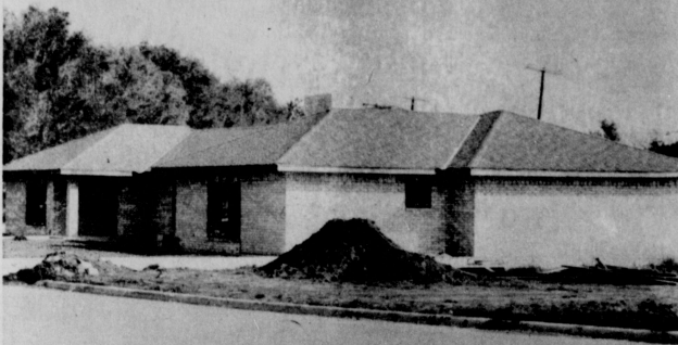
Spearman is still growing as shown here with the construction of another new home.
