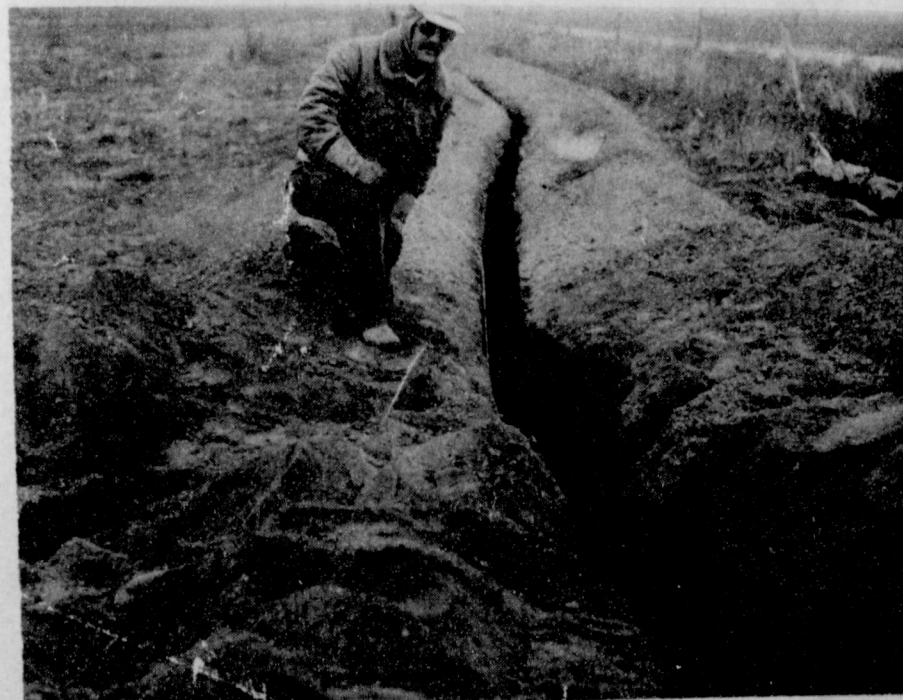
A REA man buries the lines at the end of the Spearman airport system. Our thanks to the Electric companies for their help at the new airport.
