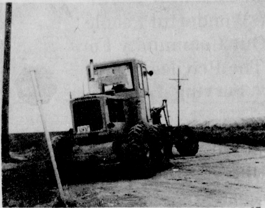
Jr. Lusby motor-grader prepares to start work on new airport for Spearman.
