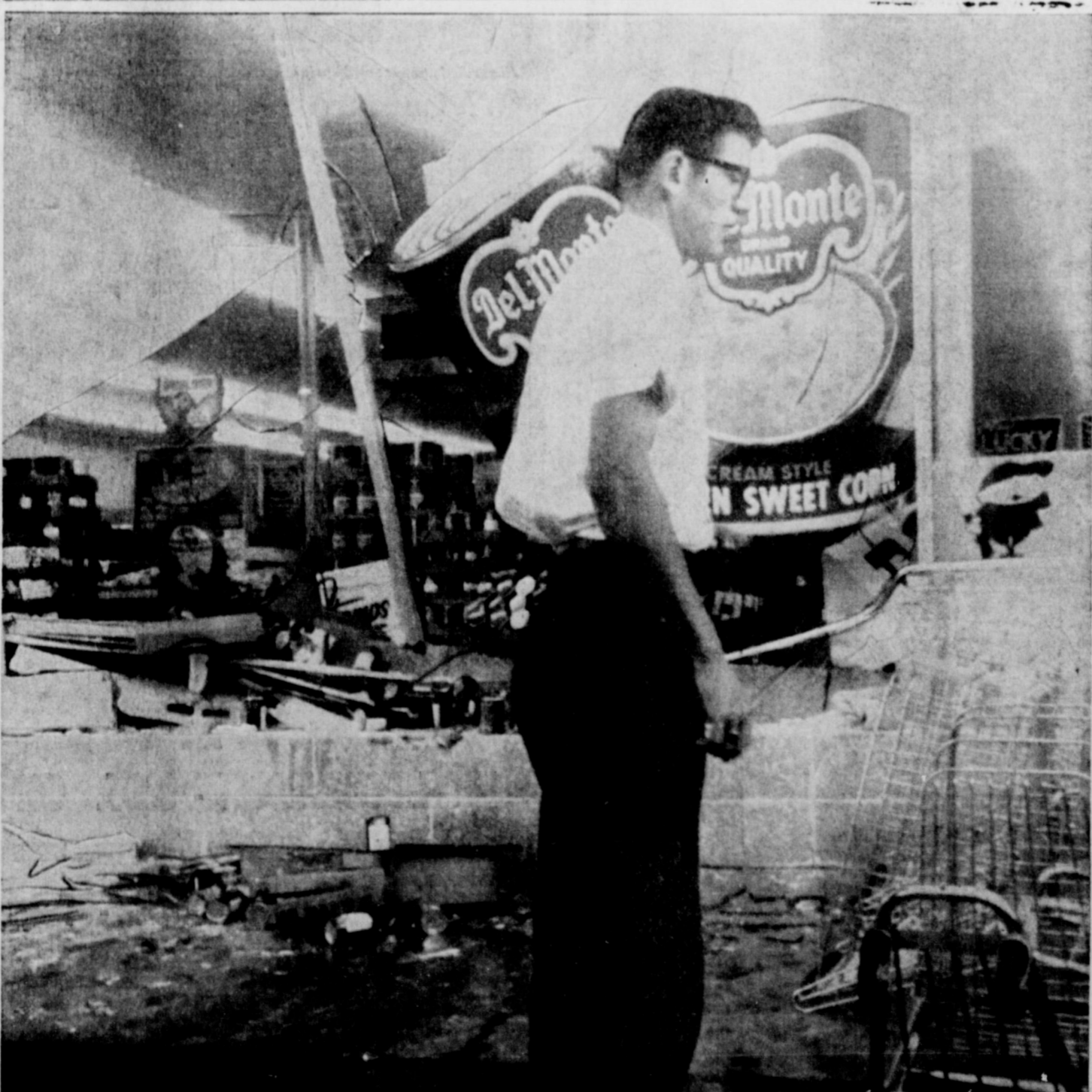
JERRY FRYE, Ideal Food Store Mgr. looks over the damage. This huge gapping hole in Ideal's store front was caused Tuesday evening by a run-away auto driven
