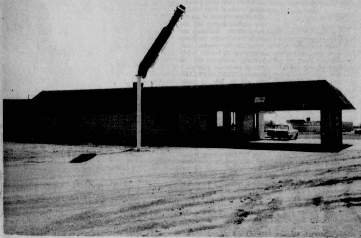
The Best Western sign at the Nursanickel Motel in Spearman was holding by one bolt, as the high wind of Monday and Tuesday almost ripped the sign down. The awning at the steak garden cafe was ripped apart and blown away during the wind storm. As we go to press today (Wd.) it is raining and sleeting!
