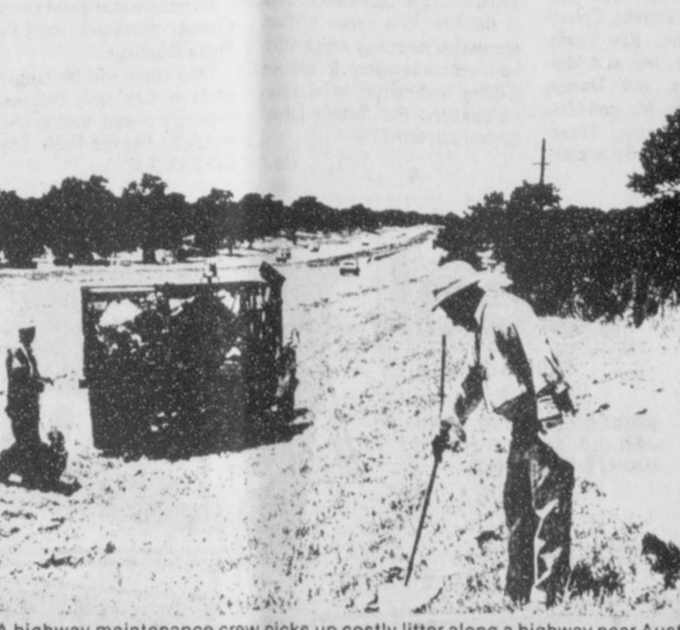
A highway maintenance crew picks up costly litter along a highway near Austin. Statewide, litter pick up expenses amounted to $10.3 million during fiscal 1980, a record high.
