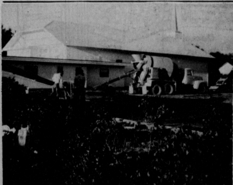
Construction has begun on the new addition to the Union Church. Pictured above is Preston Smith and Archie Smith as they pour the foundation for the 60' x 100' Pamtex Metal Building. To date, the foundation and plumbing have been completed.
