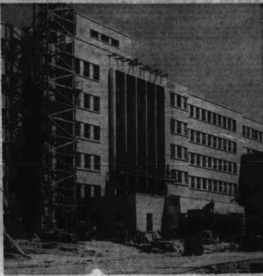
DRESSING THE FRONT — Workers have been putting touches to the trim which will dress the front of the graceful Veterans Administration hospital here. The columns, towering for five stories, are broken by bright, heavyweight aluminum panels, immediately below the entrance is being finished in granite. Front doors will be glass with aluminum trim. The project now is more than 80 per cent complete. Inside masonry and plastering are being pressed, and construction is marked for the auxiliary structures. (Jack M. Haynes Photo)
