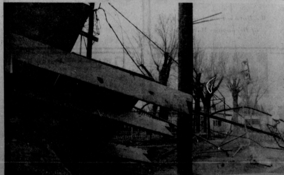
This is part of the little league park and city buildings down town Lefors. Note the lights twisted. We first thought this to be the football field.
