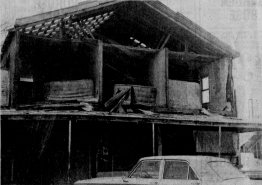
A down town building in Lefors. It was really unbelievable that more were not killed.
