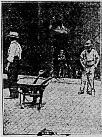
Granite Blocks Laid and Ramped — Maintenance Cost of This Kind of Pavement is Less Than That of Any Other Kind.
