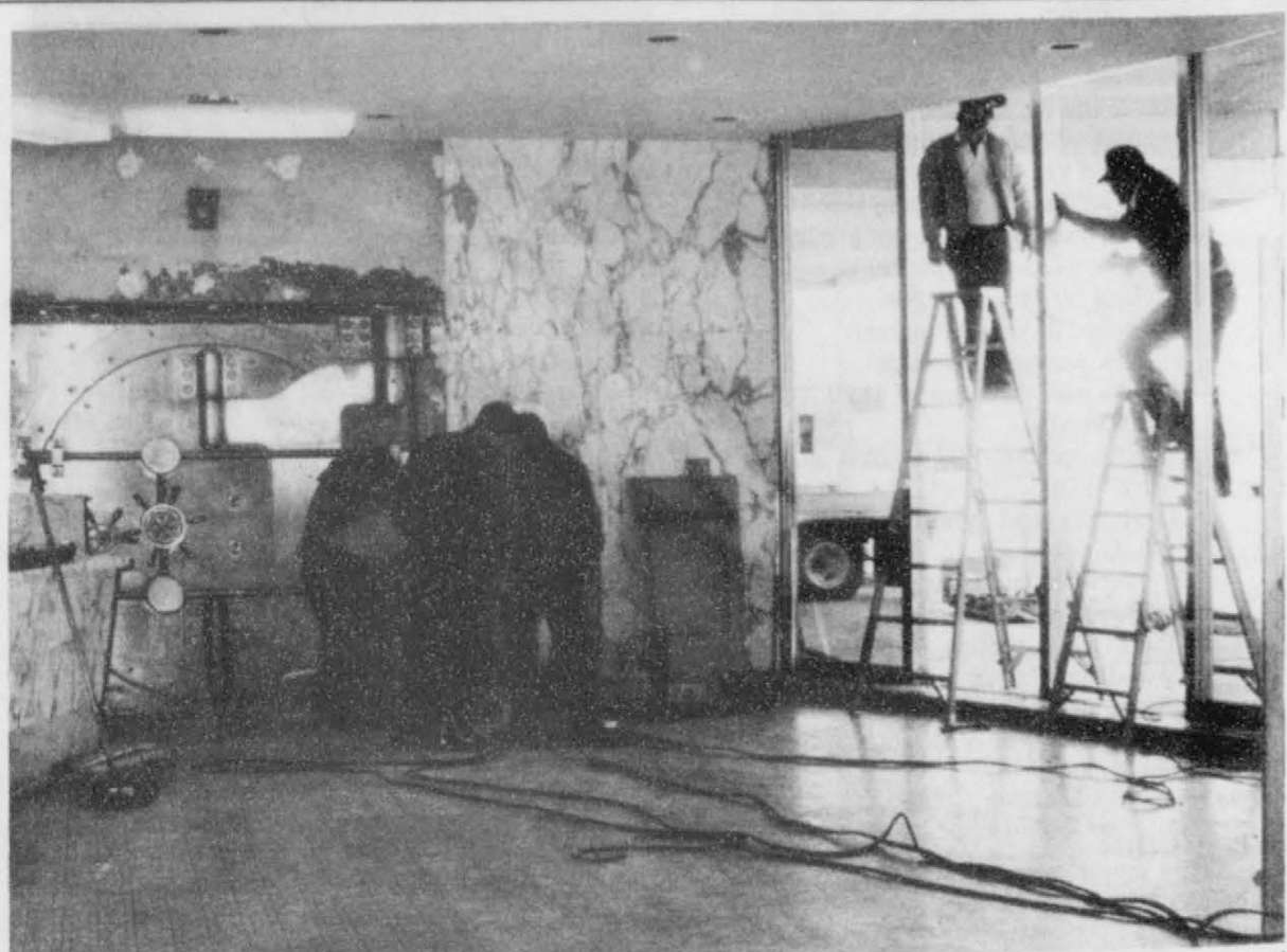
The 28,000 pound vault door was moved from the old First State Bank building to their new home this week. Workers above right, prepare to make way for the large door.
