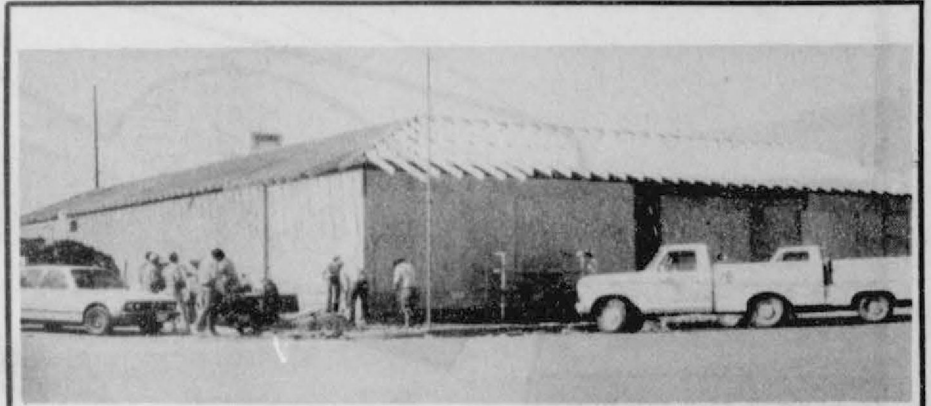
The beautiful new hip roof takes shape on the Brock Building located between the Lyric Theatre and the Post Office on Main
