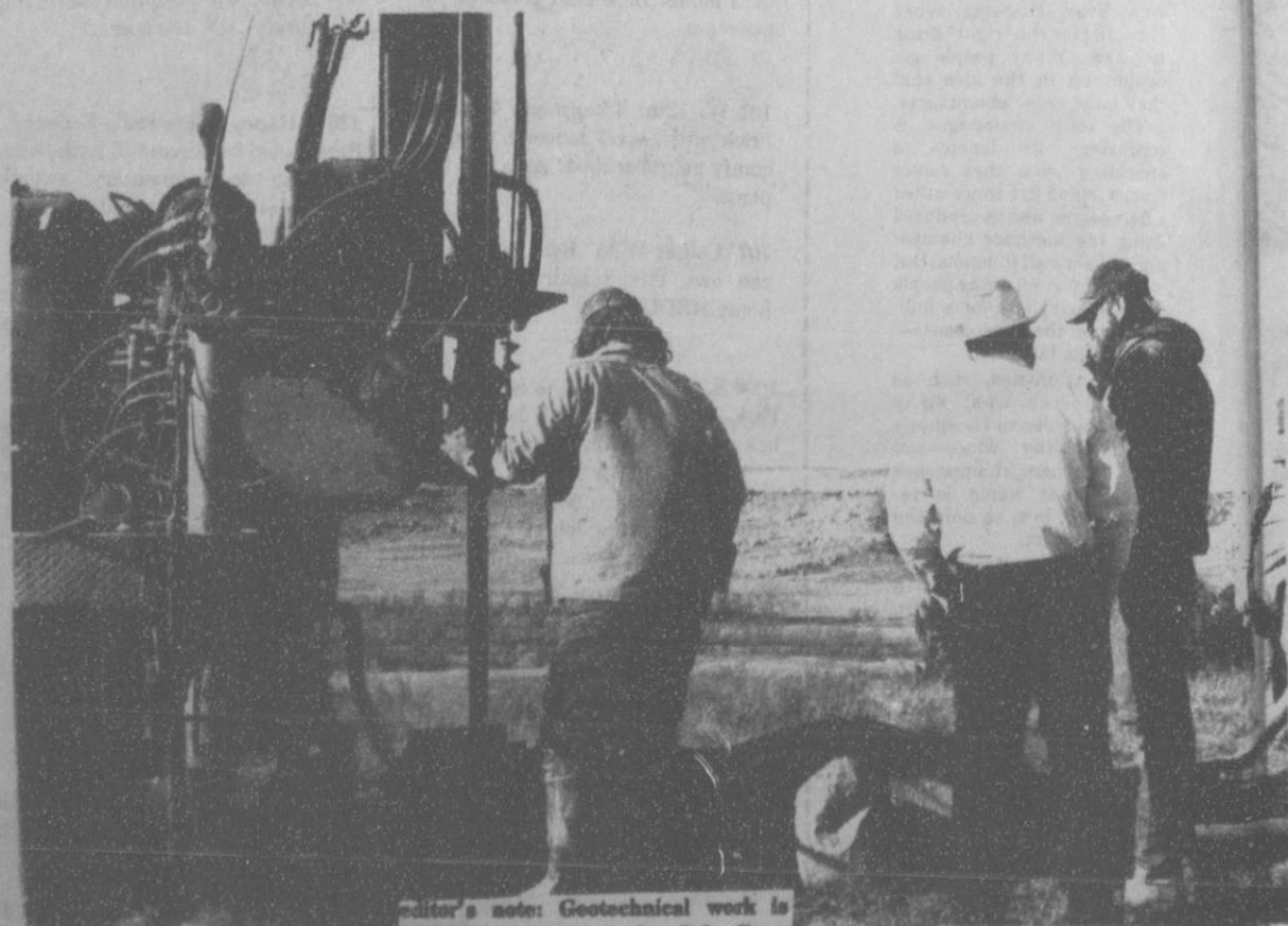
editor's note: Geotechnical work is now in progress at the Palo Duro Reservoir site.
